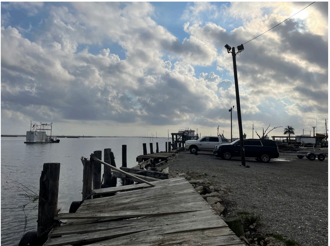
Figure 7: Pointe-aux-Chenes Marina Pier Erosion
