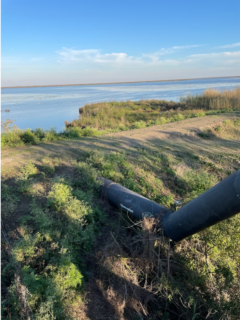
Figure 11: Woven into the marshlands, bayou, and open waters of Pointe-au-Chien are clues to the role the petrochemical industry plays. This is a pipeline photographed by the author (2022).
