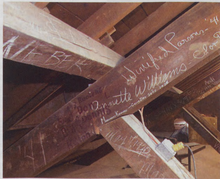
EARLY GRAFFITI: Workers renovating Kauke Hall found generations of student signatures, such as a few here from the Class of 1941, on the massive roof trusses. Matt Dilyard photo.
