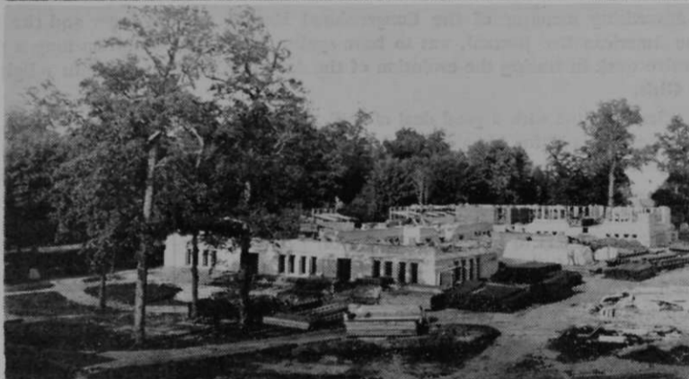
At the top is the west half of present library building. At the bottom is shown the construction work on the basement of Kauke Hall. Henrietta Street is to the left.
