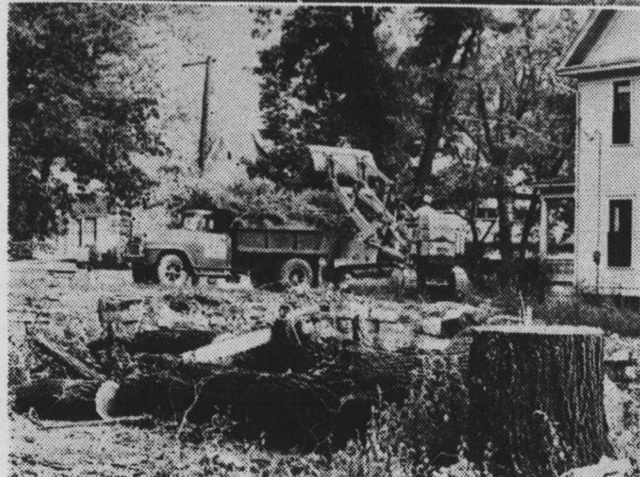
HALF A HOUSE awaits demolition to clear space for men's dorms. Below, clearing away Livingstone remains precedes Church House "ground-breaking."
